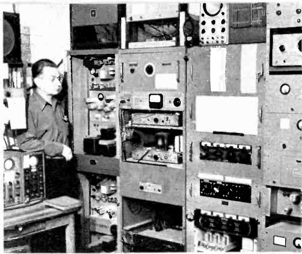
Chief engineer Perry Osborn is shown with equipment installed at Alpine, New Jersey. Multiplex modulators put several broadcasts on one carrier. Columbia University photos
