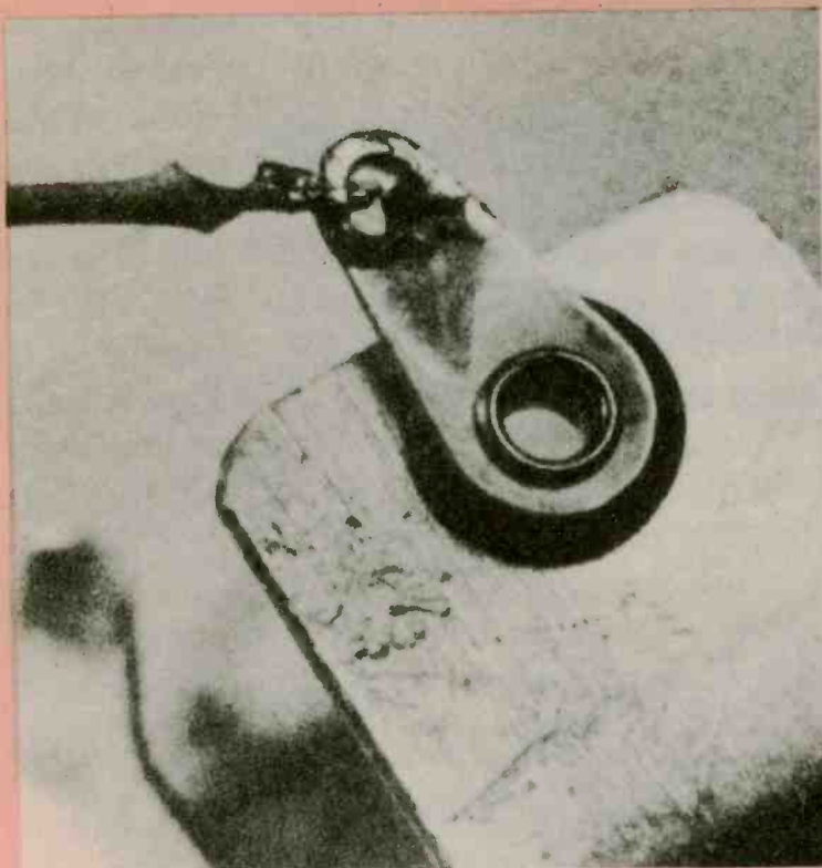
This photo a poorly soldered joint. It can break almost any time, whenever the wire is moved or flexed.
