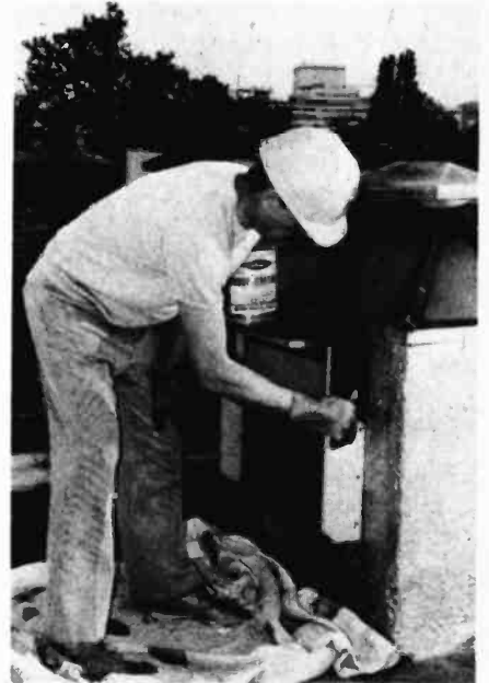
A rain shield prevents water leaks. Slope the top and paint the outer surface with roof patch material to seal all watertight.
