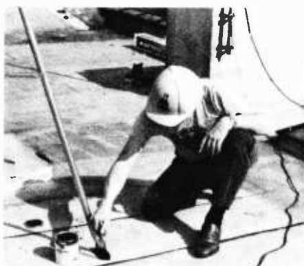
Put roofing compound over the tightened screws to keep them secure and leakproof.
