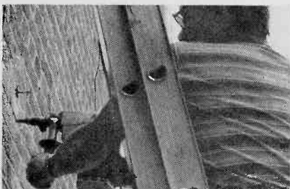
Fig. 7. While a saber saw can be used to cut through a frame outer wall, something a lot heavier is needed for brick. You can hack away at the brick with a cold chisel and sledge, but a few dollars spent to rent an electric hammer (with chisel bit) will let you bust out the wall in minutes. Note the screw sticking through the pilot hole, used to center the duct circle scribed with chalk.
