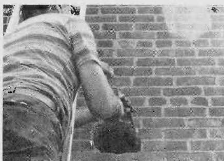
Fig. 8. The final trim is done by hand with a cold chisel and small sledge. The sheet metal duct should just slide through the hole without bends or a force fit. Chip away small bits of brick until the duct can slide in and out easily.
