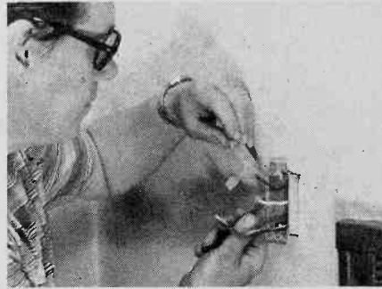
Fig. 6. Before cutting the outer wall and mounting the fan unit, install all the necessary electrical wiring. While you can use a simple on-off switch, a multi-speed selector switch or variable speed control can be a great help when you want to move air slowly, in small quantities.
