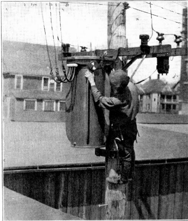
Fig. 124. This photo shows a pole type transformer and the method of making primary and secondary connections. Also note the thermometer temperature indicator near the hand of the electrician.
