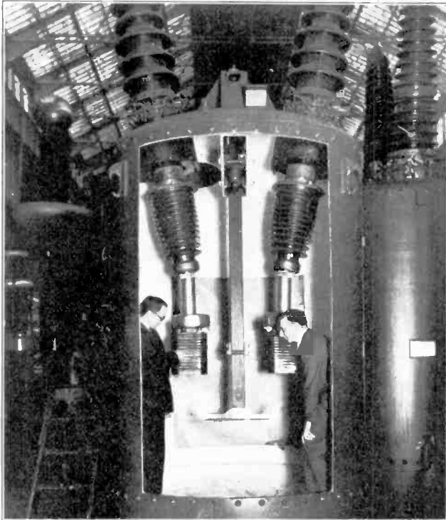
Fig. 428-B. This unique photograph clearly shows the inside of a large high-voltage oil switch equipped with Deion grids on the stationary contacts. Note the size of the contacts, insulators, and tanks required for handling the currents of high-voltage power lines. Courtesy of Westinghouse Elec. & Mfg. Co.
