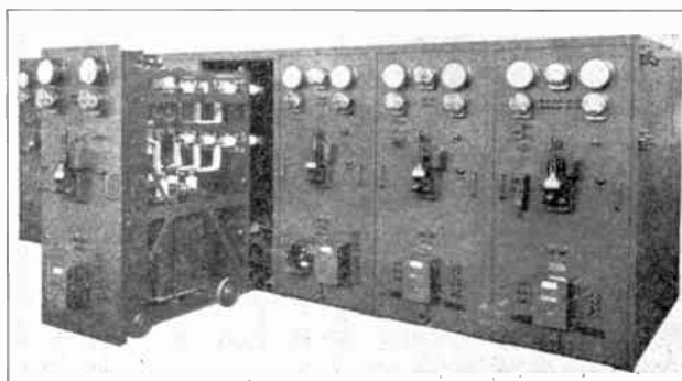
Fig. 418. View of truck-type switchboard showing one section removed to allow repairs or adjustments to be conveniently and safely made. Boards of this type are very popular in modern industrial plants as well as in certain power plants and substations. (Courtesy of G. E. Company.)
