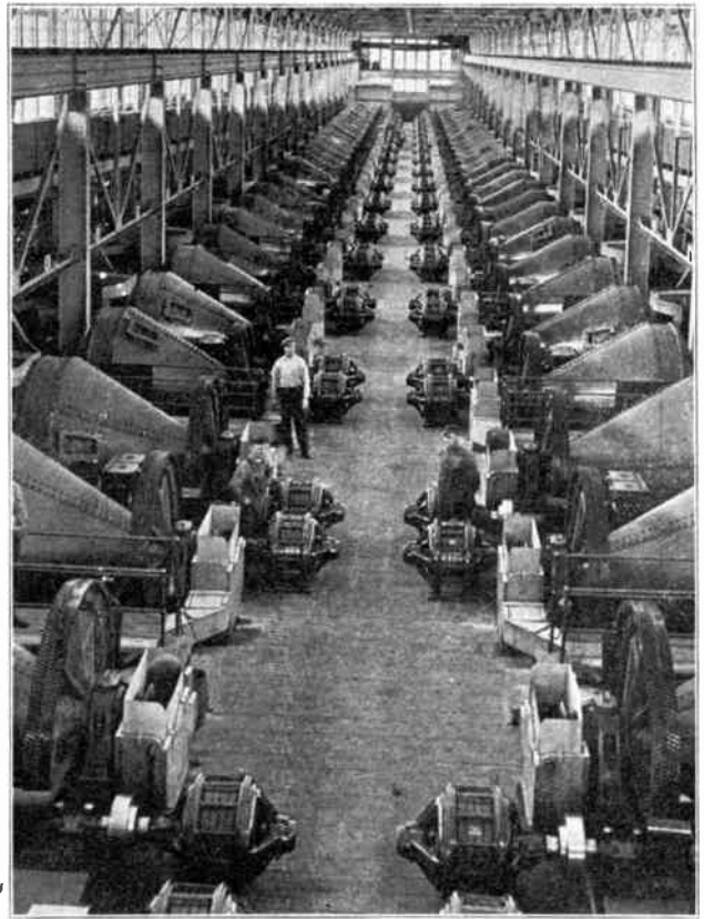
Fig. 475. This photo shows an installation of A. C. motors in a copper mill. Hundreds of thousands of motors in thousands of electrified factories and plants require the services of trained electrical maintenance men.
