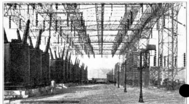
Fig. 414. View of large oil switches and lightning arresters underneath the bus and switching structure of a 220,000-volt outdoor substation. (Courtesy of Philadelphia Electric Company.)
