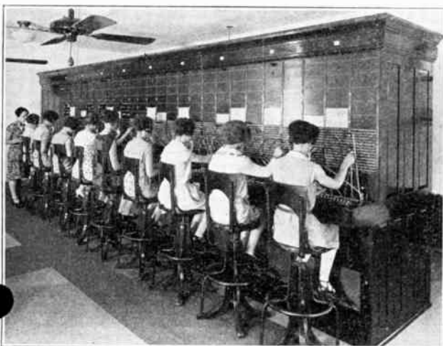
Fig. 147-F. This photograph shows a section of a large manual telephone exchange. Each operator controls a section of the board with its respective plugs and jacks.
