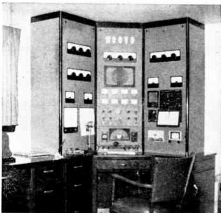
This neat "built-in" installation features separate finals and exciters for each band, along with room for receiver, frequency meter, oscilloscope, Q multiplier and v.h.f. converter. All units are mounted on the three large panels; the panels are hinged at the bottom so that they can be lowered for service work on the individual units. A common power supply is used, and band-changing consists of turning on the filaments in the desired r.f. section. (W90VO, Sturgeon Bay, Wisc.)
