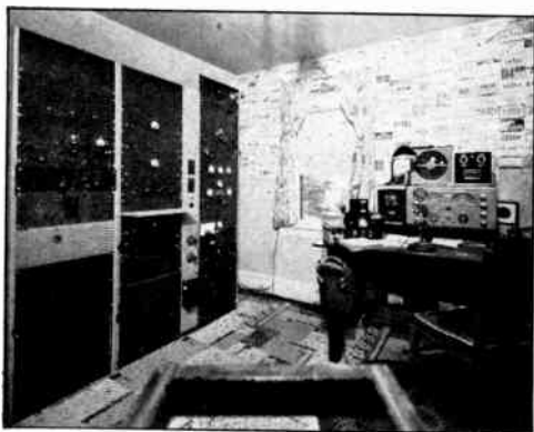
A high-powered station in a room with enough space to locate the transmitters along one wall and the operating table along another. Note the convenient location of the control switches, and the receiver raised above the table. (WICII, Worcester, Mass.)
