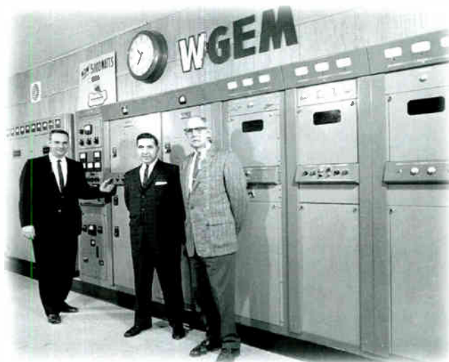
A new Gates transmitter was installed for WGEM AM in 1962. (left to right) Frank Loughlin, WGEM chief engineer; Joe Bonansinga, WGEM general manager; and Thomas C. Oakley, president of Quincy Broadcasting Company.
