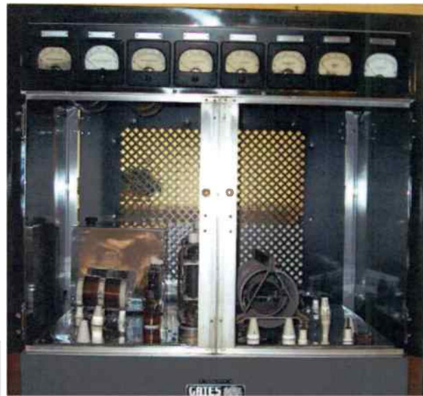
Front View Showing Meters
