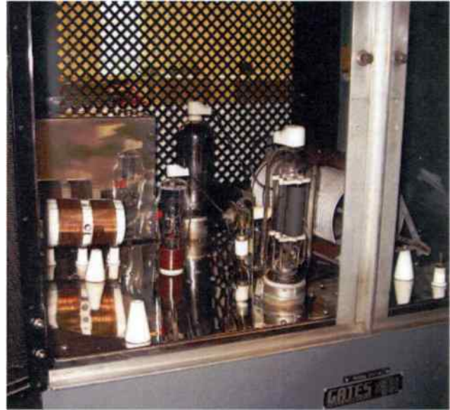
R.F. Deck Showing 810's
