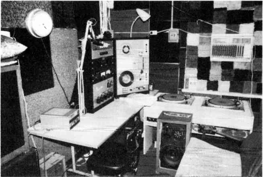
Emergency Control Room near transmitters
