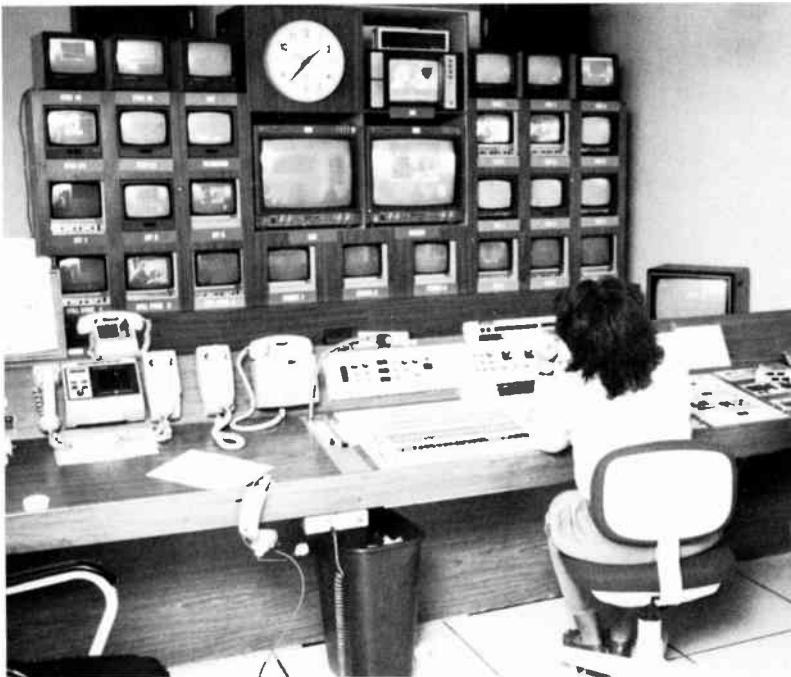
The control room at WTNH. (WTNH 8, New Haven)
