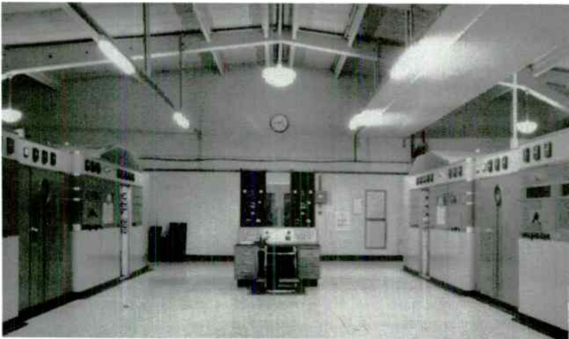
Figure 14.2 RCA transmitters at Woofferton from 1943 to 1970
