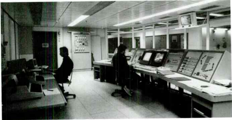
Figure 22.3 The control room at the Pori SW station
