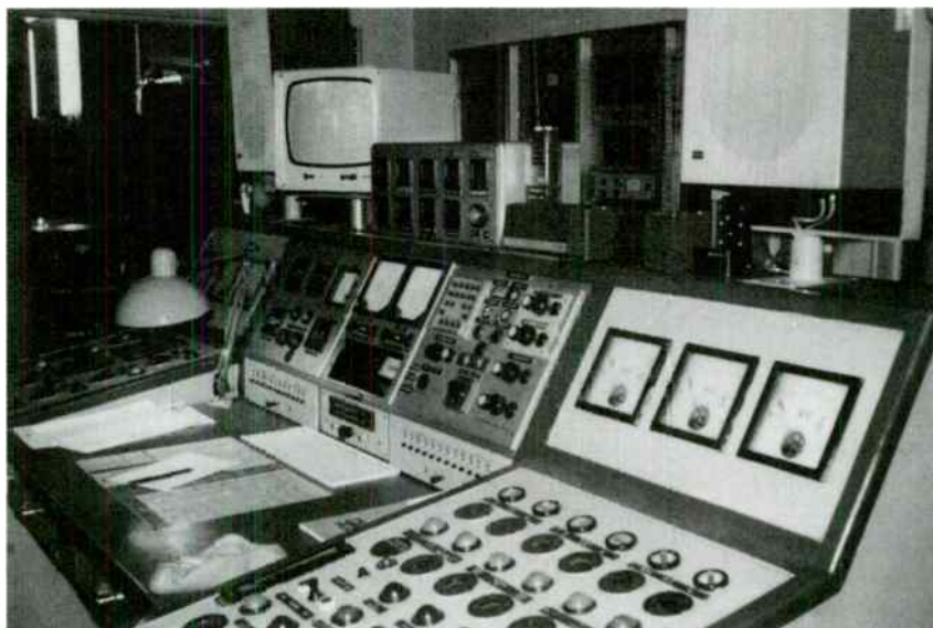
Figure 21.3 RIAS Berlin control room at Britzer Damm SW station, 1989
