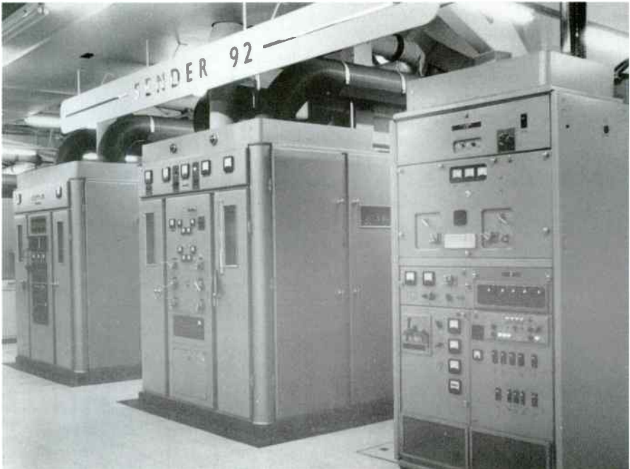
Figure 20.1 Marconi BD-272 transmitters installed at the Woofferton VOA relay station in 1963
