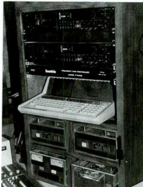
FIGURE 9.18 Equipment rack containing cassette tape machines, car- tridge machines, and computer termi- nal. Rack mounted for convenience and ease of handling. Courtesy WMJX-FM.
