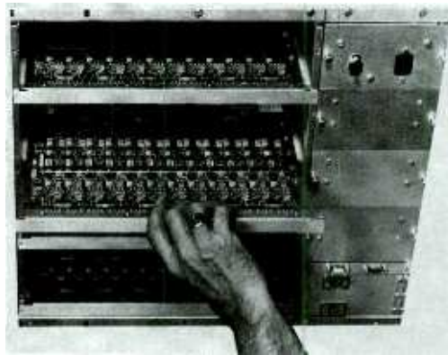
FIGURE 10.21 The luxury of solid-state electronics—pull out the bad, put in the good. Courtesy IGM.
