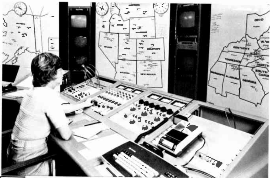
Figure 12-9 Satellite control centers can select and transmit programming to any number of selected geographical regions.
