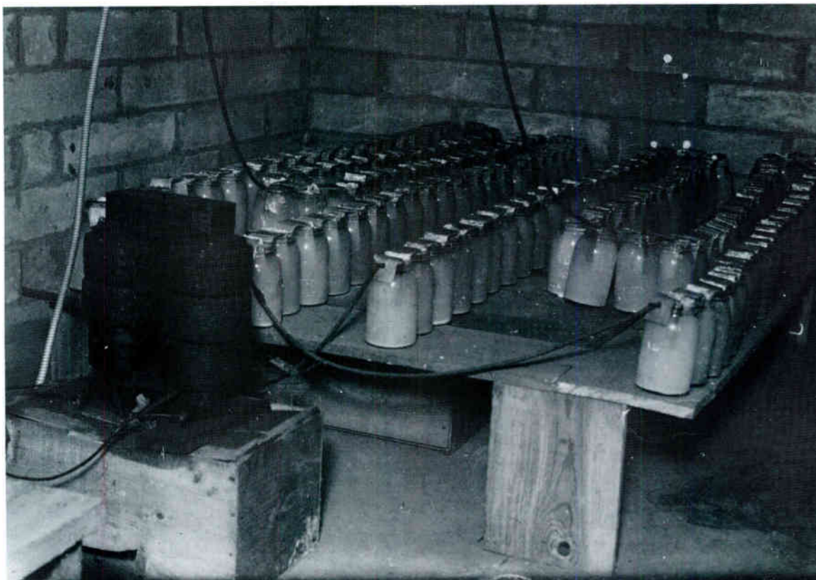
The transmitter's Leyden jar power supply in the basement.
