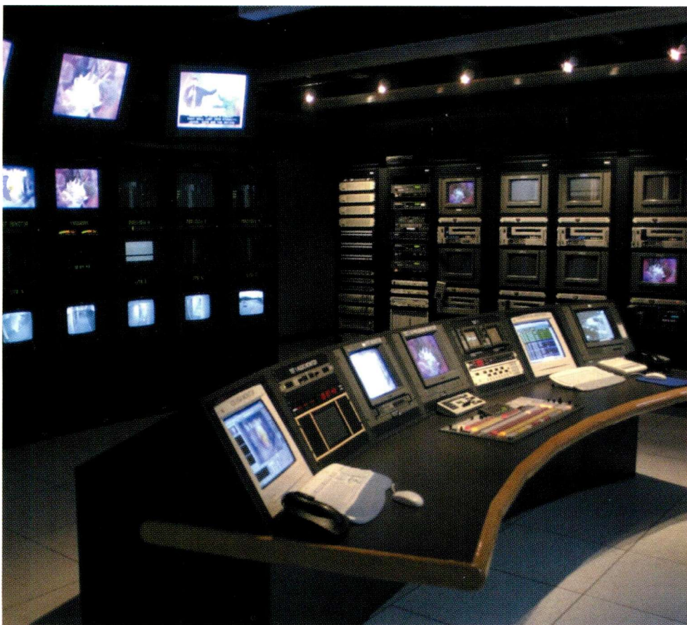
Master control room at The Word Network – Southfield, Michigan.
