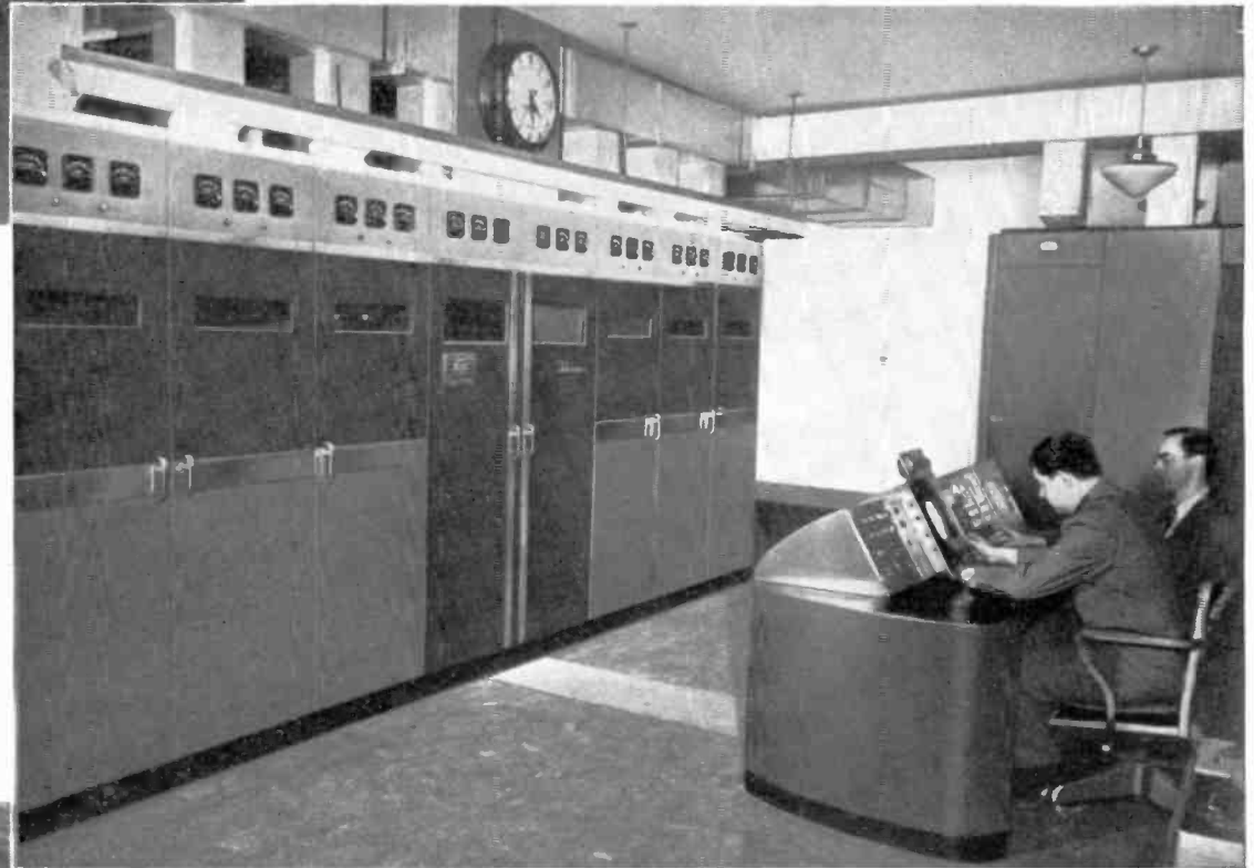
WJZ-TV's Empire State transmitter room is completely RCA-equipped. It includes a 5-kw transmitter (plus 2.5 kw for FM sound), a 500-watt stand-by transmitter, control console, antenna diplexer, vestigial side-band filter, dummy load.
