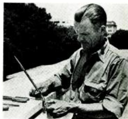
Lightning-arrester installation on the roof of the White House recently completed by the George E. Thompson Co., Minneapolis, which features use of 1/2" lightning conductor cable from all television and radio antenna fed to 1/2" copper ground rod 10' long.
