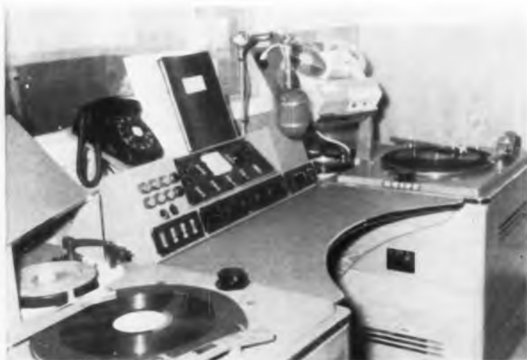
Fig. 1: The control room set-up which is used by the combo man in small stations.
