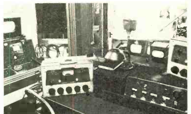
Fig. 4: Split booth isolates audio operation from video, cuts down important ambient noise
