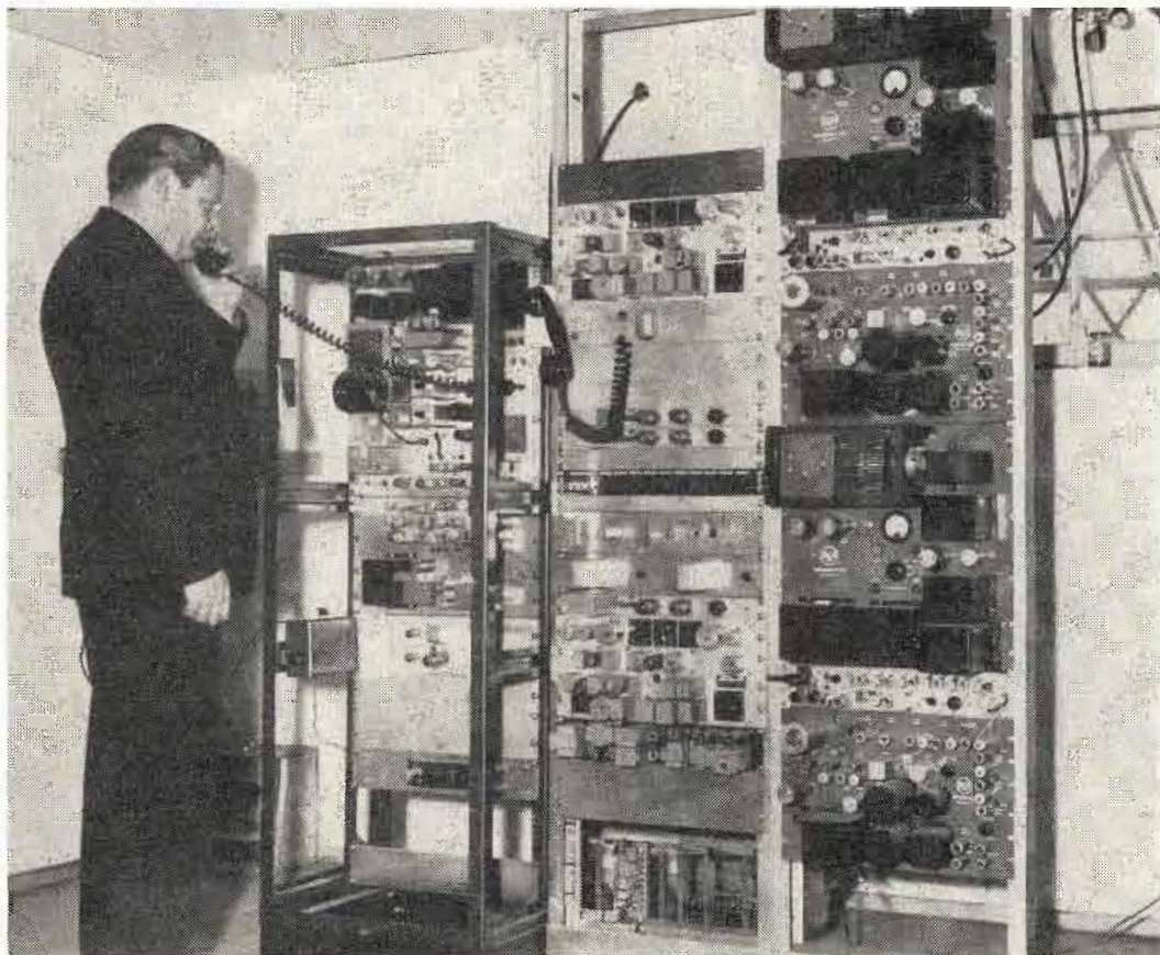
Fig. 2: Terminal station where VHF ties into the microwave system. Shown in temporary housing are (l to r) VHF transmitter and receiver, multiple channeling equipment, and microwave relay rack
