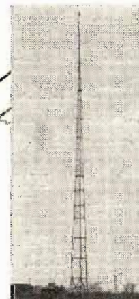
WUSJ-FM, Lockport, N. Y., Truscon Self-Supporting Tower, 135 feet high and supporting a GE 4-bay FM antenna 42 feet high. Overall height 177 feet.
