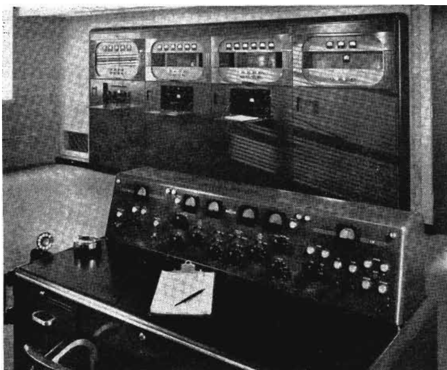
Control console for the two transmitters is a single unit located with a clear view of both. It contains frequency and modulation monitors and VI meters for each transmitter
