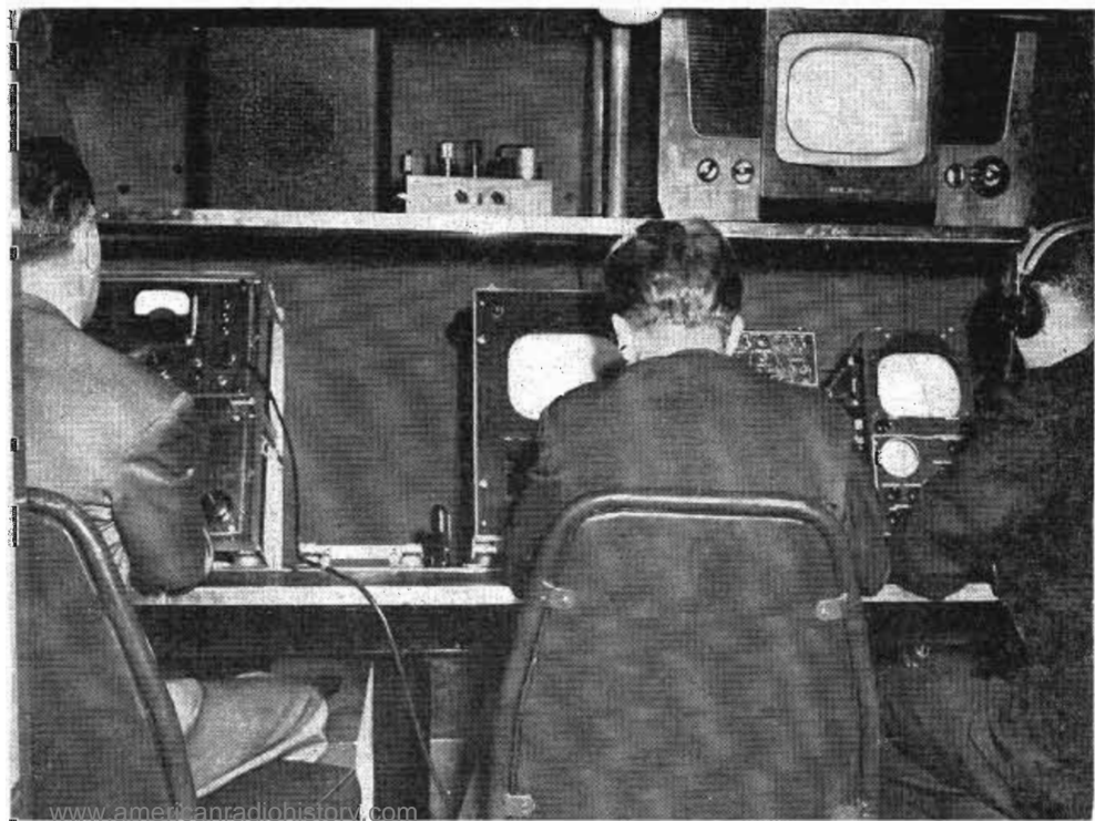
Remote mixer and preamplifier (l); master monitor (center); camera control unit (right)
