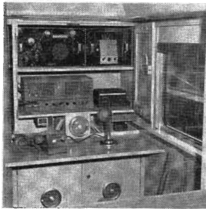
Arrangement of the Western Electric radio equipment in the General Motors "Train of Tomorrow", permitting passengers to call anywhere while train is en route
