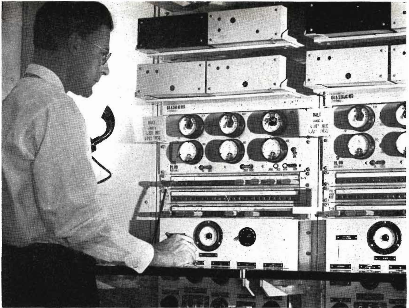
At Philadelphia, a testboard man answers as an electronic watchman calls attention to conditions on one of the coaxial systems to Baltimore and Washington.
