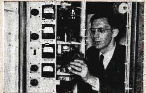
WALL-MOUNTED UNITS afford easy access to all tubes and wiring. Rear doors further increase ease of reaching all components. Illustration above shows portion of the aural transmitter's r-f driver unit.
