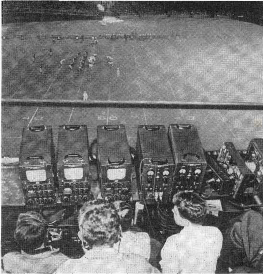
FIG. 2—Control equipment for a dual camera chain set-up as used for a field pickup
