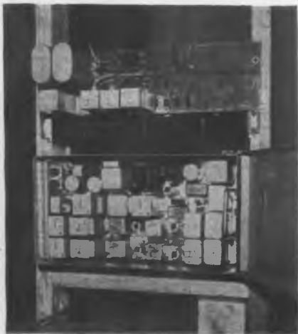
Terminal equipment for wired radio system which REA and Southern Bell Telephone have installed to provide subscribers with local telephone service by carrier
