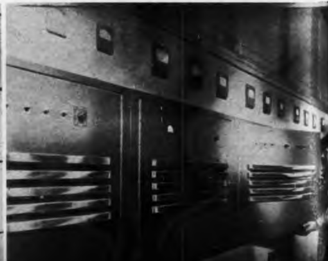
Another view of the same transmitter, a model 50HG, which is now broadcasting the Voice of the United Nations
