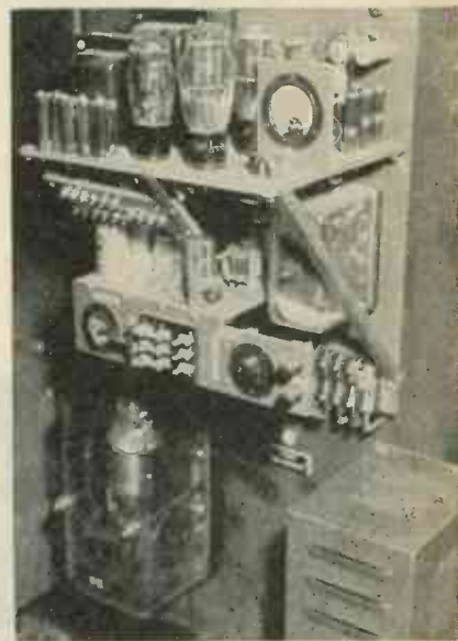
Amplifiers and relays of generator vibration control
