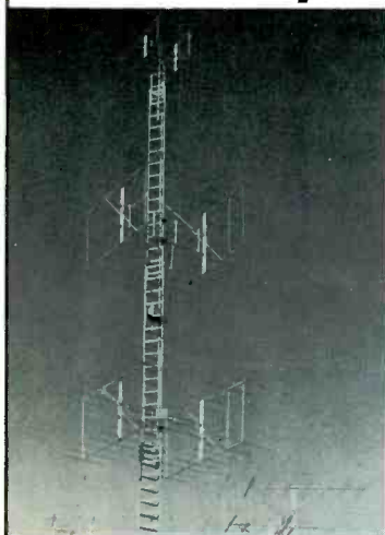
A Typical SITCO Installation
