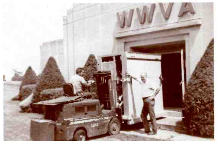
In July 1969, when the new 50,000 watt transmitter was installed at the WWVA St. Clairsville transmitter site, it took men and machines to handle the big job.
