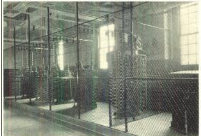
High voltage transformers increase 2,300 volts alternating current to 20,000 volts.
