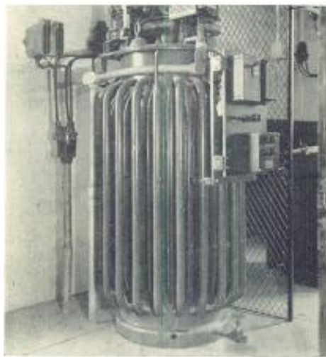
Automatic induction regulator keeping constant the voltage on the 100-kilowatt tubes.
