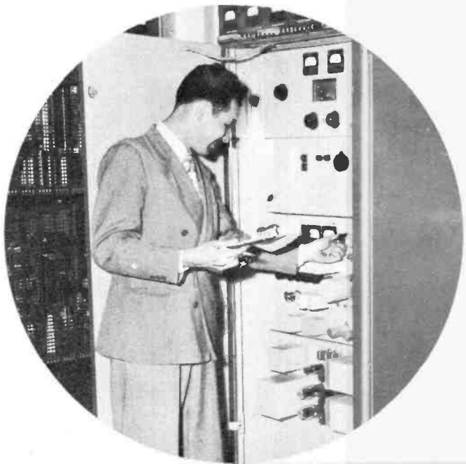
Willy Trofumik makes a minute adjustment on the Frequency modulation transmitter, recording the reading on the log.
