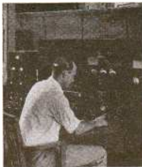
The control board at the transmitter connected with six circuits to the control board at the studios.
