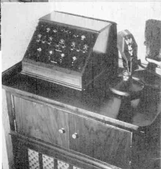
Announcer's control panel, below, located in each studio showing control buttons and signal lights.
