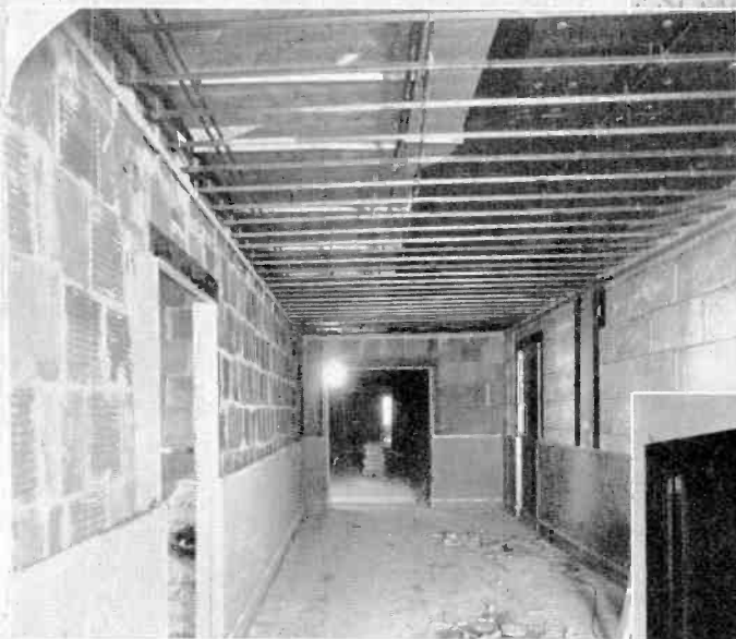
View from control room into studio "B" showing construction of the sound-proof partitions. Three panes of glass are used. The two panes facing the studio are slanted to disperse sound waves and avoid echoes.
