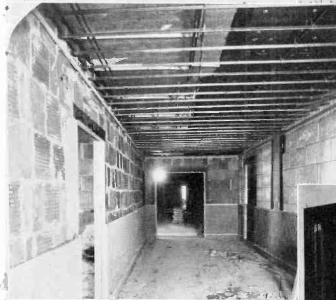
View from control room into studio "B" showing construction of the sound-proof partitions. Three panels of glass are used. The two panels facing the studio are slanted to disperse sound waves and avoid echoes.
