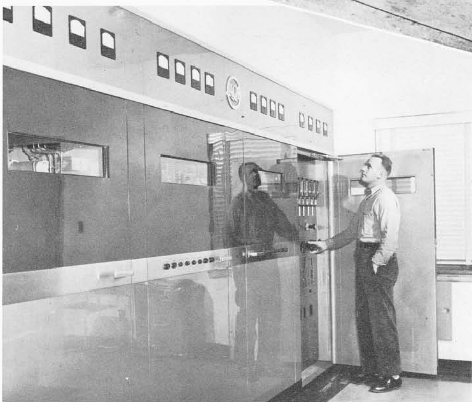
Ed Mohr and a portion of the Control Panel of the WKOW Transmitter.
