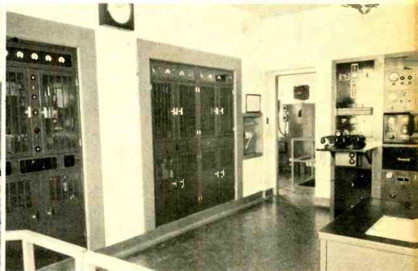
The operations room of WIBW's 5000 watt transmitter. The shield enclosing the high-voltage apparatus is along the left wall, with the operations panel at rear right. WIBW engineers must exercise extreme care in working in the vicinity of the tremendous electrical current.
