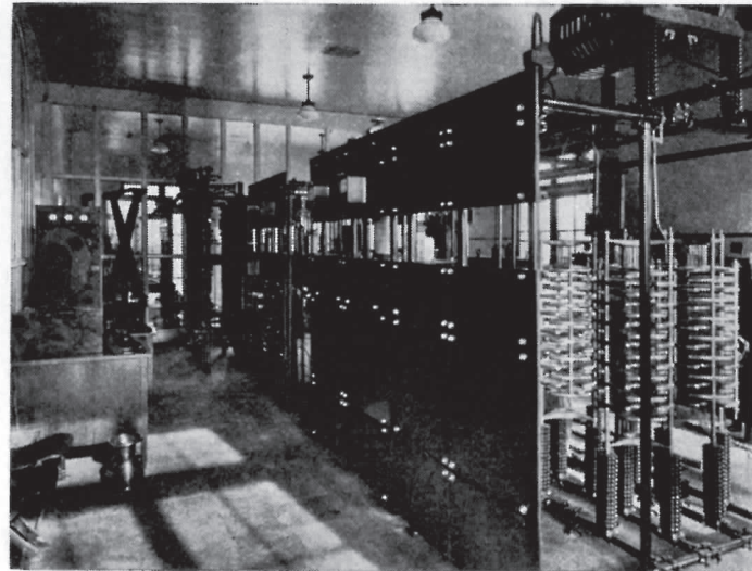
The W-G-N transmitter, a powerful 15-kilowatt at Elgin, Illinois. Every radio word and note of music travels up and down behind these panels before leaping from the aerial, over the hills and far away to your radio horn.
