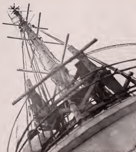
SIGHT-AND-SOUND AERIAL —New antenna atop Empire State Building, New York City, for Television Station W N B T and FM Station W EAF -FM.
