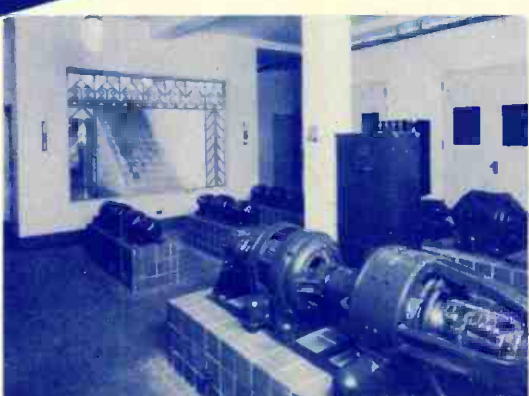
Power machinery for developing KOA's 50,000 watts.
