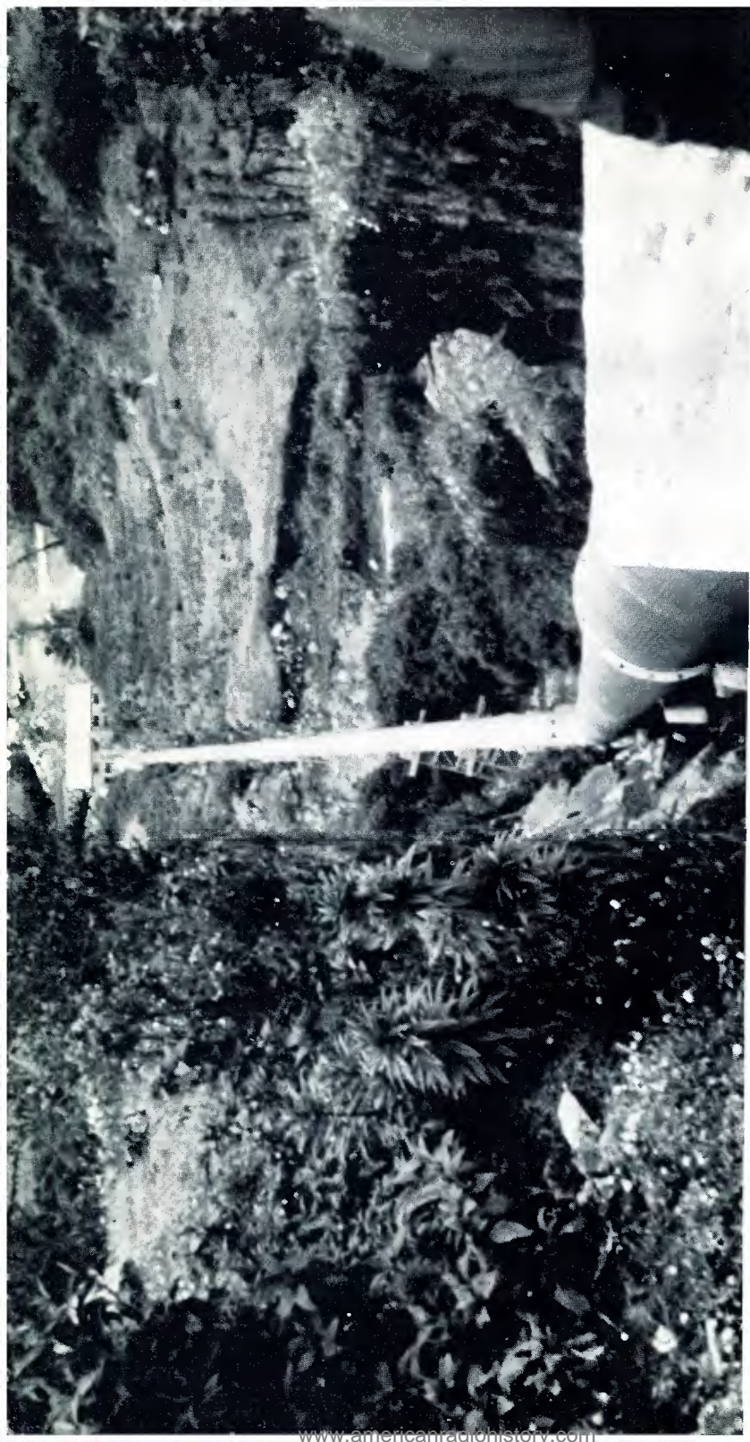
Penstock leading to hydro-electric building where the power for HCJB's transmitters is generated in Papallacta, Ecuador.
