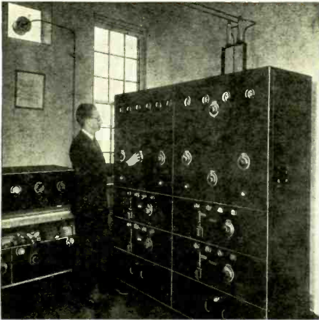
Radio frequency exciter equipment recently remodeled for W3XAL. Carl Dietsch at the controls. (Fig. 1.)
