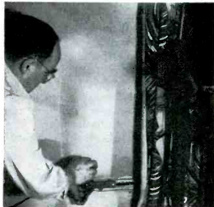
Fig. 9c. Installation of an absorption-type wavetrapp on a baseboard.
