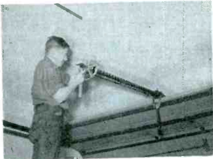
Fig. 6. Driving the pulley on to the end of the worm. Notice the position of the angle iron over head, and that the partly open door supports the weight of the worm.
