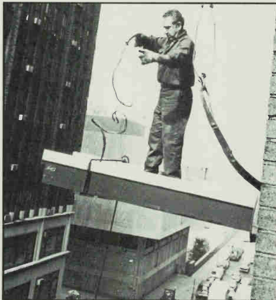
A rigger nonchalantly stands on the 20' steel camera track, seven stories above the ground, as it's being guided into its new home.
