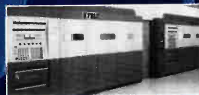
100 kW SW Transmitters
