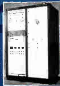
11 kW FM Transmitter
