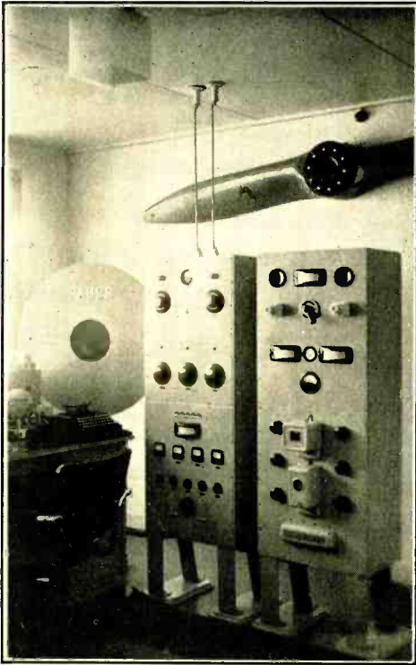
The unusually neat and commercial appearing installation at PAΦBB which was in use until Dutch equipment was interned by the authorities as a precautionary measure.
