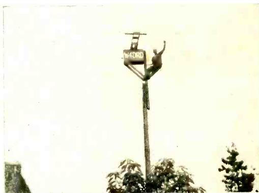
When the rotating head is placed atop the pole and the radiators are attached, the installation looks like this.
